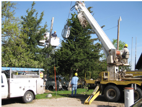
Electrical work underway getting camp ready for summer. It takes a complex infrastructure to maintain the quality of services at Moses Merrill Camp & Conference Center.
